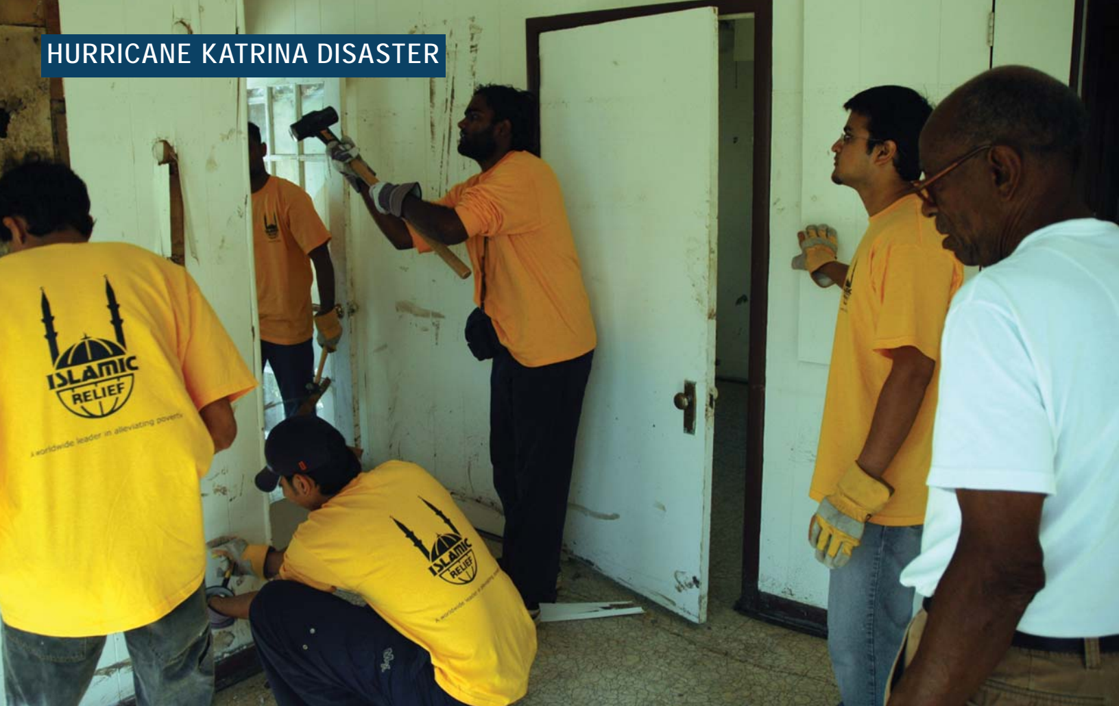
Islamic Relief volunteers gut out a Hurricane Katrina damaged home in Biloxi, Mississippi as the homeowner looks on.
