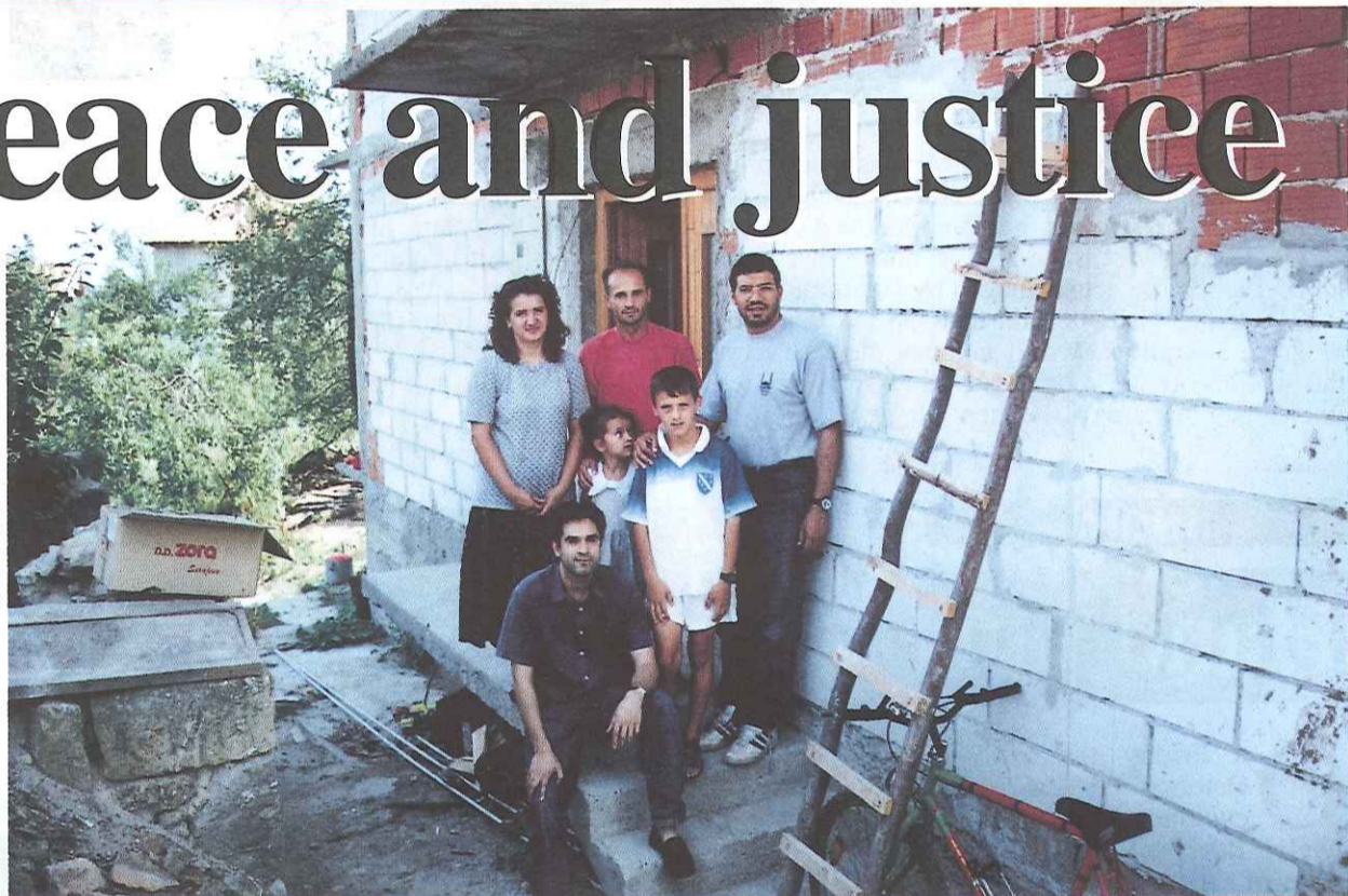
Mirsad Okic and his family have returned to their home in the Dulici village of Zvornik municipality. Their house is undergoing extensive repairs with help from Islamic Relief staff Sikander Ali and Mostafa Osman
