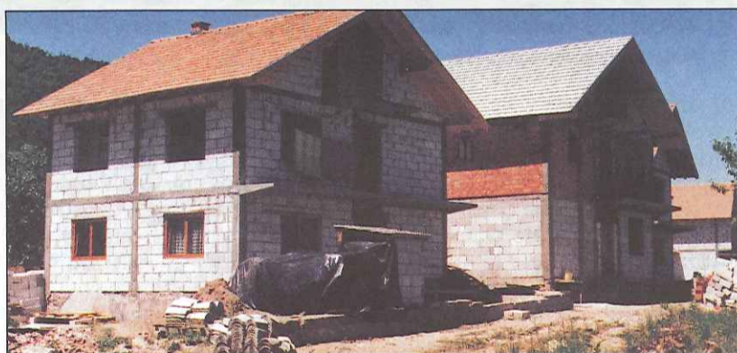
Houses repaired by Islamic Relief, in the Hajdaravici village of Zvornik municipality
